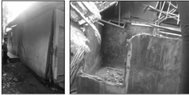
Figure 1. Condition of the roofs and walls of houses due to landslides. (Source: personal documentation).
